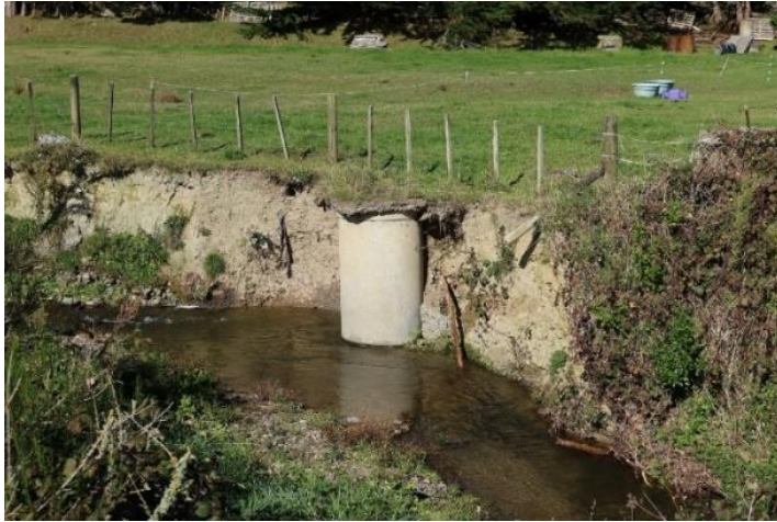
Figure 3. Exposed man pipe.
