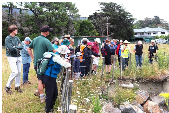
Checking out the erosion. 28/01/2024.
